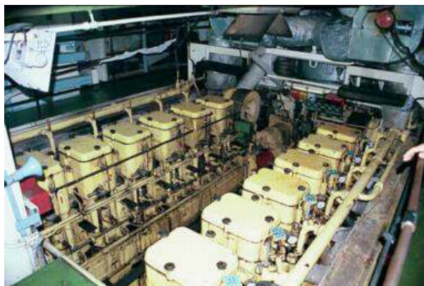
Figure 18 – The Engine Room
